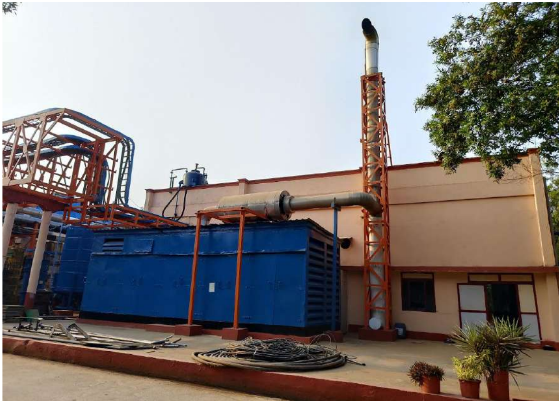
Photographs of Diesel Generator sets in the plant
